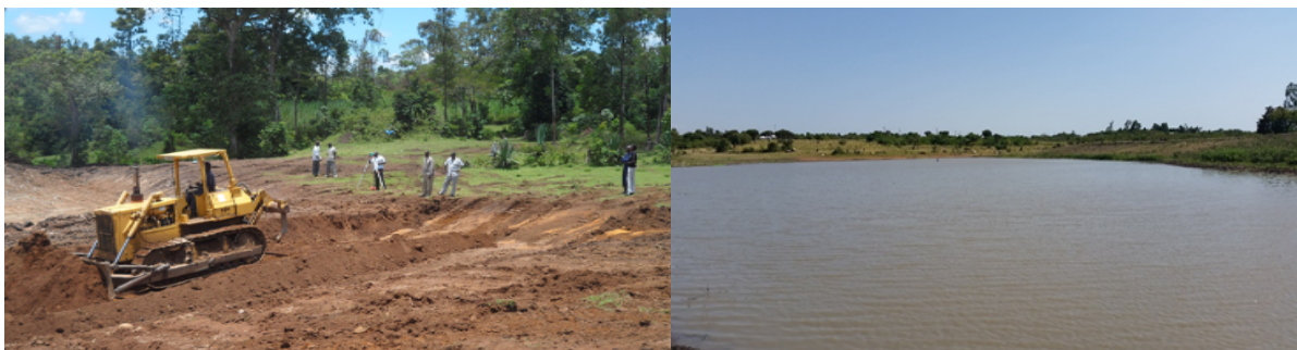
A bull dozer from Agricultural Mechanization Services, undertaking construction of Okenge II water pan and the completed Okenge II water pan in Nyatike Sub County.
