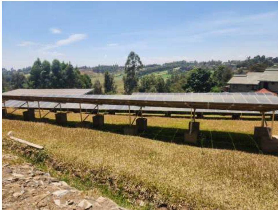
Figure 1 Solar mini grid in Ondiri Water Scheme that will hold a total capacity of 338kWp
