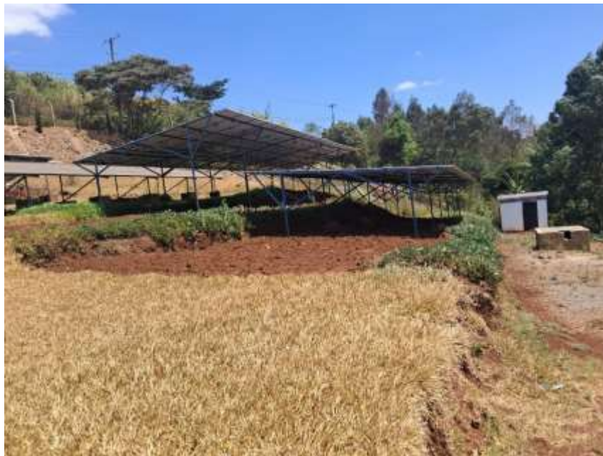
Figure 2: Solarized Borehole at Ondiri in Kikuyu that pumps 60m 3 /hr
